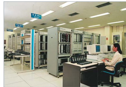
TDX (Fully Electronic Switching System) : Opening a new chapter in Korea’s communications history
